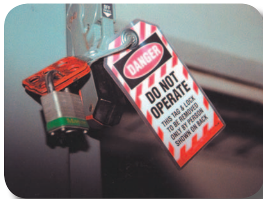
Example of Lockout/tagout used on electrical equipment
