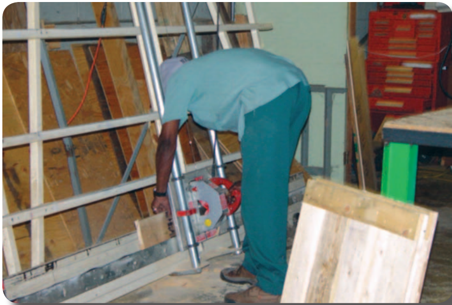
Worker in awkward posture to use saw.
