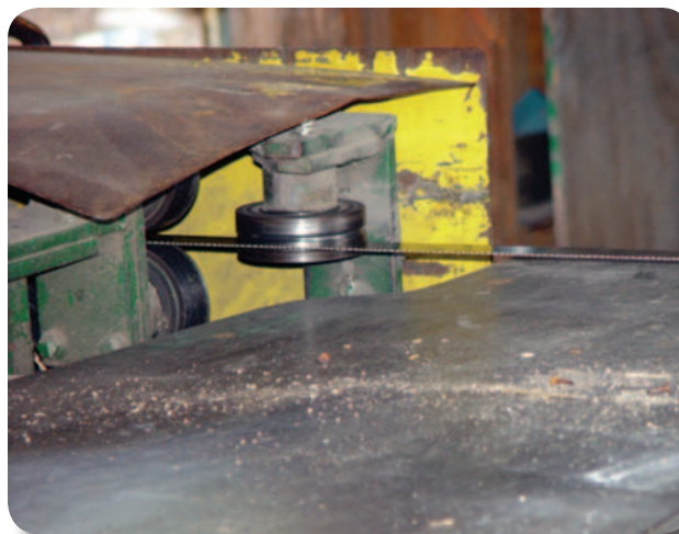
Band saw for recycling pallets that has no guarding.
