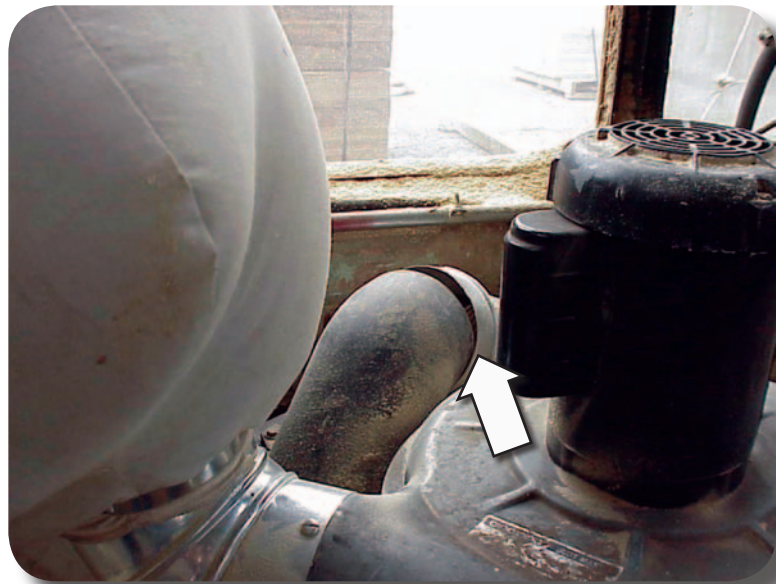
A gap in the ductwork of an exhaust system
