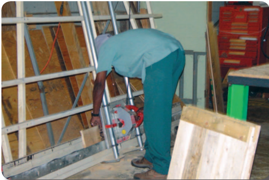
Worker in awkward posture to use saw.
