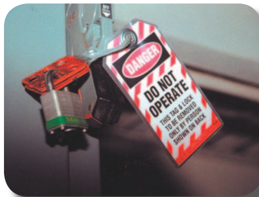
Example of Lockout/tagout used on electrical equipment
