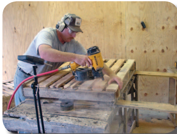
The worker's free hand is very close to the firing end of the nail gun.
