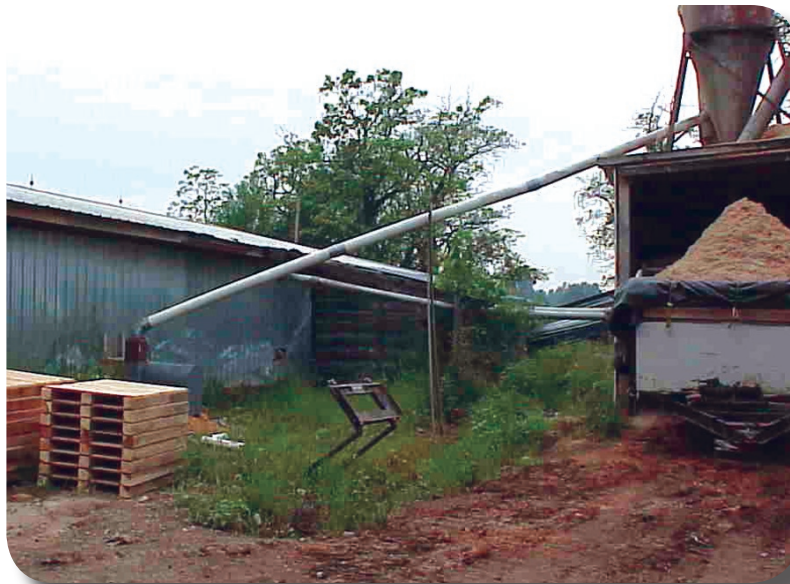
Outlet for a central exhaust system. The exhausted material is piled too high and is not protected from rain and wind.
