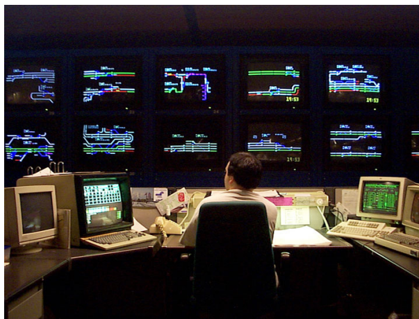
Figure 1. Modern dispatching center
