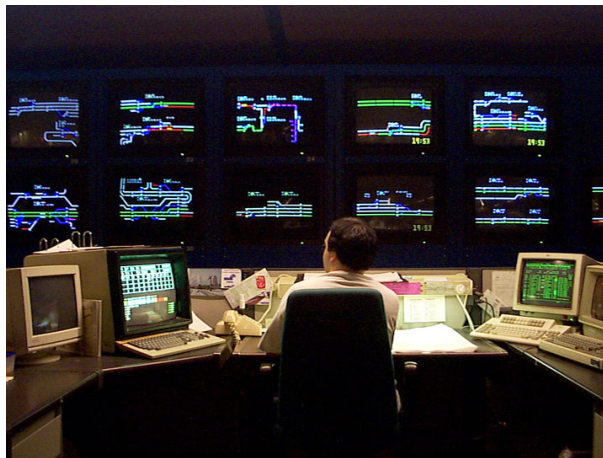
Figure 1. Modern dispatching center
