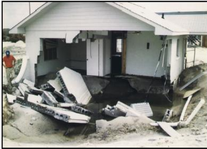
Post-storm field studies have shown that minimally compliant A Zone foundations in Coastal A Zones often fail. (Hurricane Fran)
