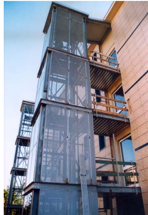
This smokeproof elevator is installed at an Italian residential facility for mobility impaired people to provide access and egress. The glass hoistway enclosure permits the fire service to determine if the elevator is in use. (courtesy CNR)
