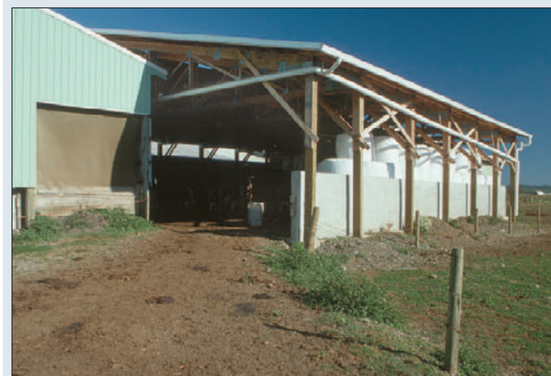
Water run-off control with the use of a gutter system at a dairy in Tillamook, Oregon. (Photo courtesy of USDA/NRCS)
