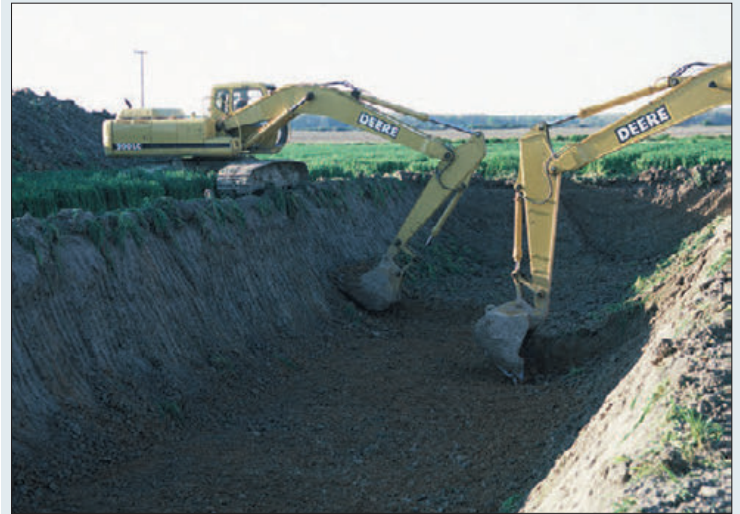
Construction of a storage pond at a farm in Lonoke County, Arkansas. (Photo courtesy of USDA/NRCS)
