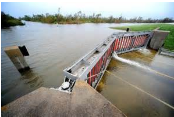
Figure 14 - Gate Controlled Diversion Structure
