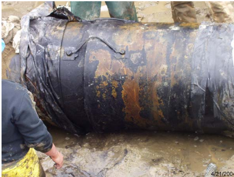
Figure 2—Surface corrosion noted underneath PE encasement
