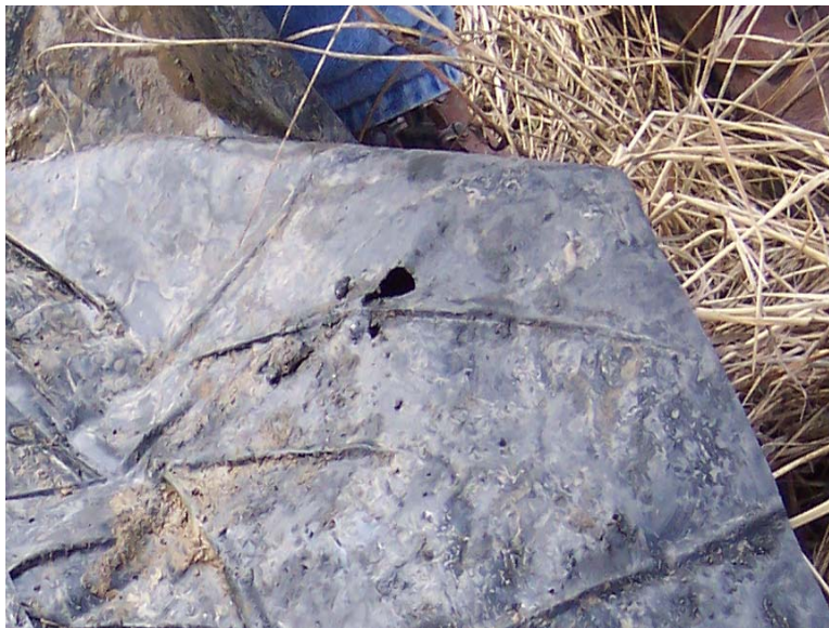
Figure 4.—Close up view of PE encasement with numerous perforations.
