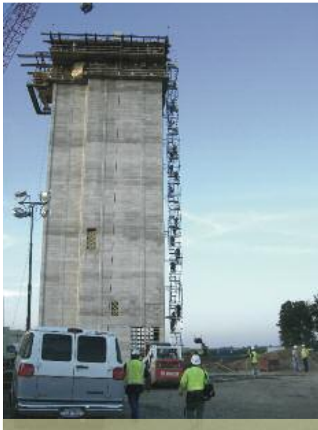
New Vision Co-op’s feed mill in Magnolia, Minn., during construction. The grain elevator at the $12.6 million facility is expected to open by November, with the feed mill to be in operation by June.
