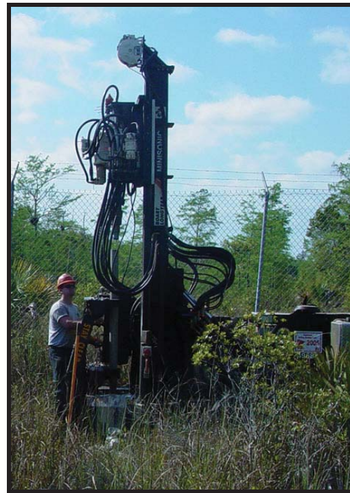
In other areas such as Big Cypress National Preserve, operators have used sonic drilling technologies to drill shotholes which eliminated drill cuttings on the surface that must later be cleaned up.
