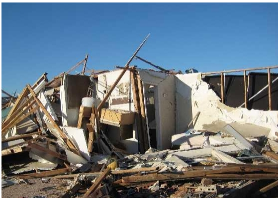
This residence has collapsed.
