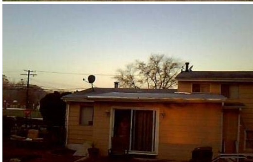
The roof on this residence has been tarp covered after it lost some shingles.
