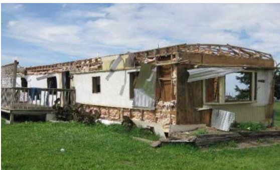
This manufactured home is missing the roof covering, and at least one wall has been compromised.
