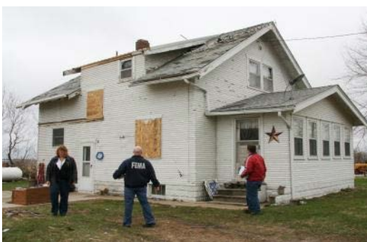
This residence has nonstructural damage to the roof and broken windows.
