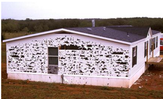
Nonstructural components of one wall have sustained damage.
