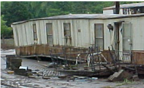
The frame of the manufactured home has been bent.
