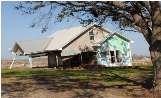
The foundation and two or more walls of this residence have failed.
