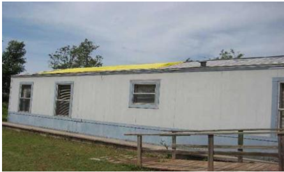
A portion of the roof has been damaged.
