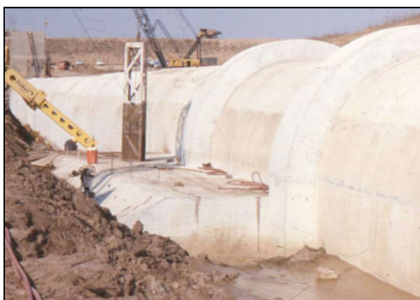
Portion of concrete plug along conduit (outlet works station 50+00 and dam station 71+50)
