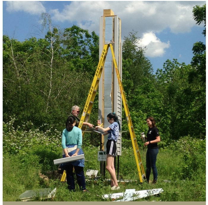
Chimney Swift tower construction at Hartrick Park in Lansing MI. Michigan Audubon
