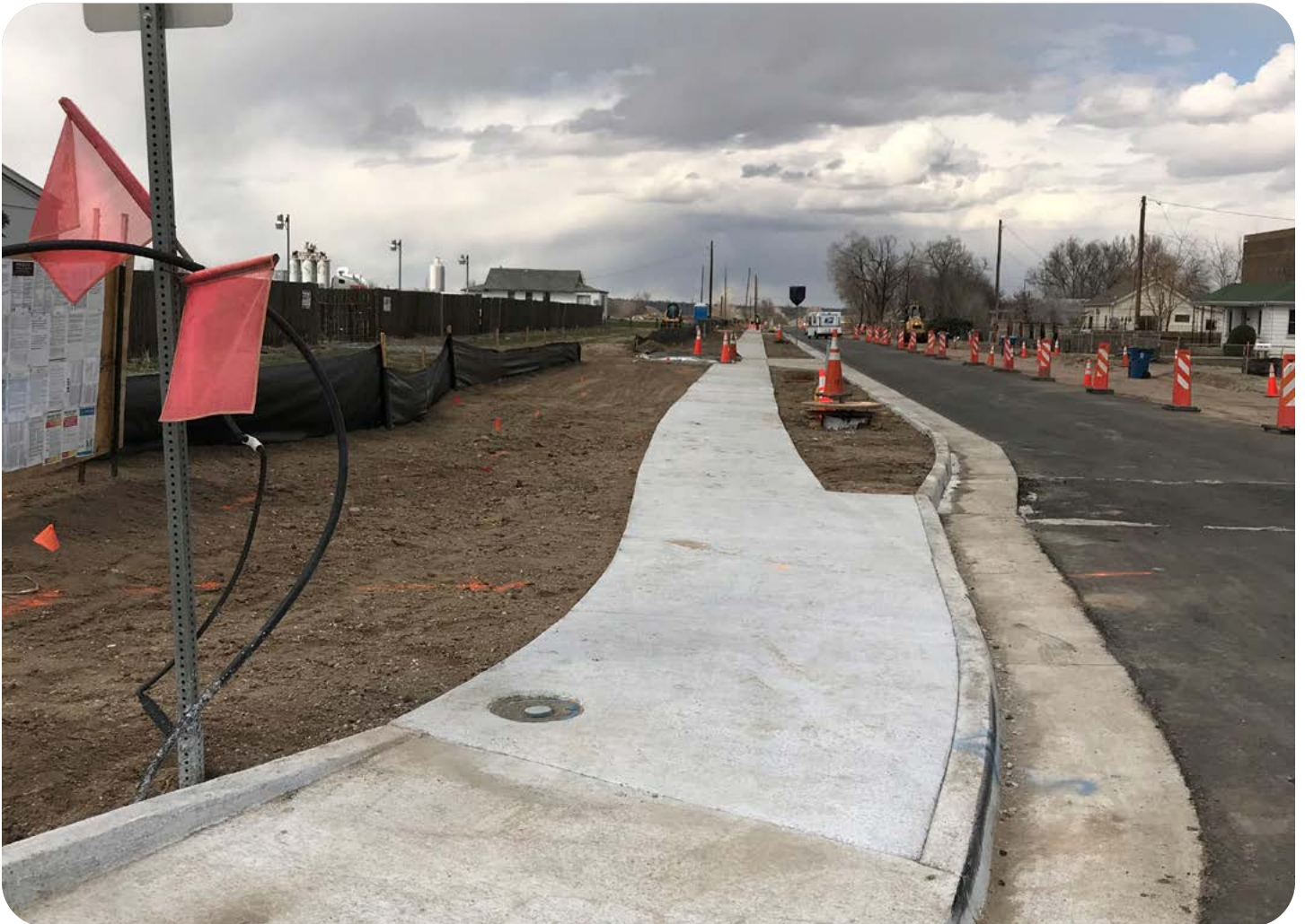
When streets and roadways are widened and reconstructed, sidewalks and curb ramps must be brought into compliance with Americans with Disabilities Act standards. Photo credit: Commerce City
