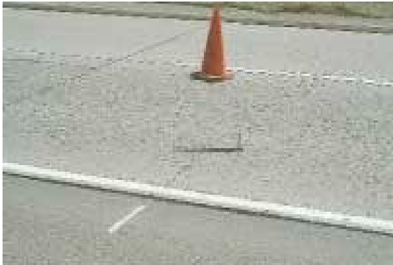
Figure 84: JCP Moderate Severity Transverse Cracking
