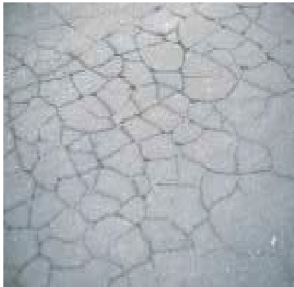
Figure 71: AC Chicken Wire/Alligator Fatigue Type Cracking
