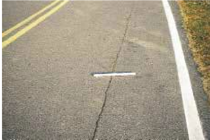
Figure 70: AC Moderate Severity Longitudinal Cracking
