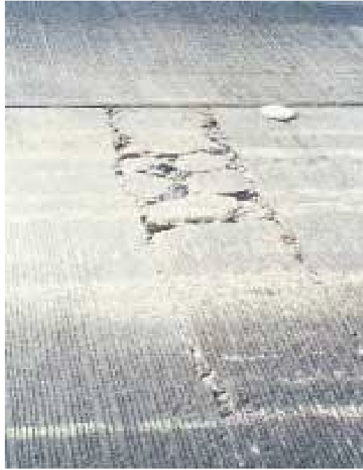
Figure 78: High Severity CRCP Punchout Cracking
