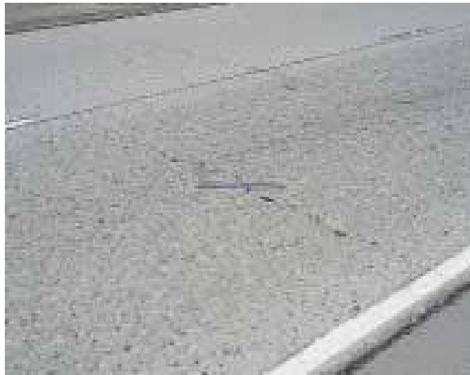
Figure 85: JCP High Severity Transverse Cracking
