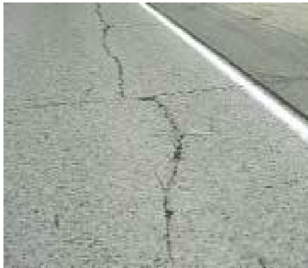
Figure 82: JCP High Severity Longitudinal Cracking
