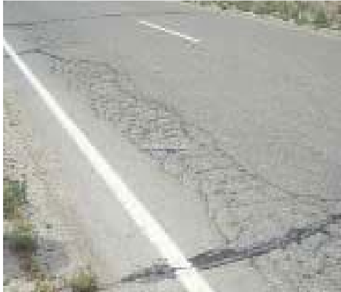
Figure 74: AC High Severity Fatigue Type Cracking
