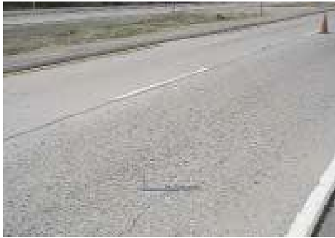
Figure 80: JCP Low Severity Longitudinal Cracking
