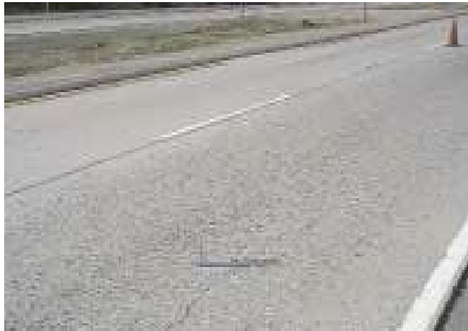
Figure 80: JCP Low Severity Longitudinal Cracking
