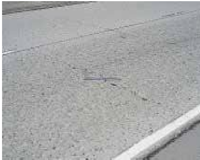
Figure 85: JCP High Severity Transverse Cracking
