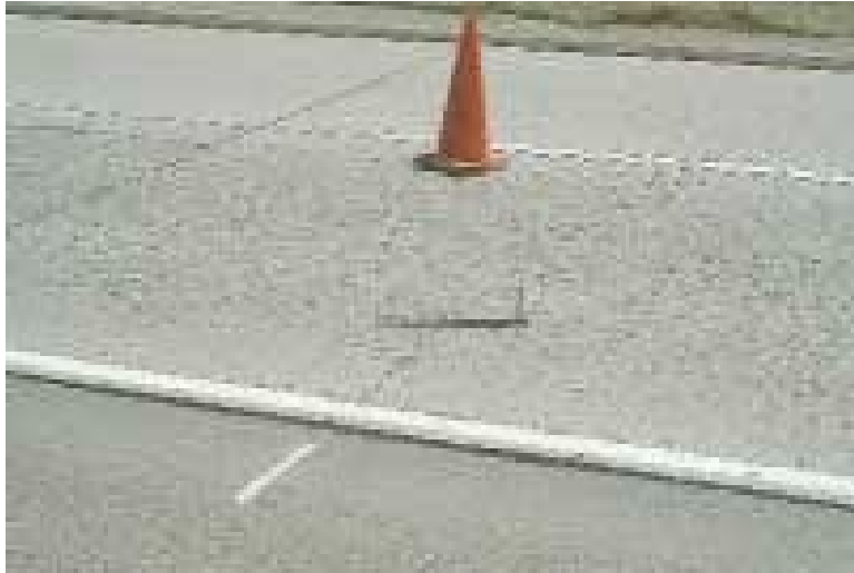
Figure 84: JCP Moderate Severity Transverse Cracking
