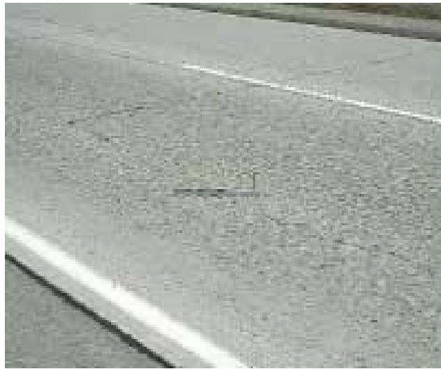
Figure 81: JCP Moderate Severity Longitudinal Cracking
