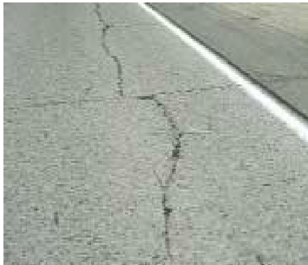
Figure 82: JCP High Severity Longitudinal Cracking
