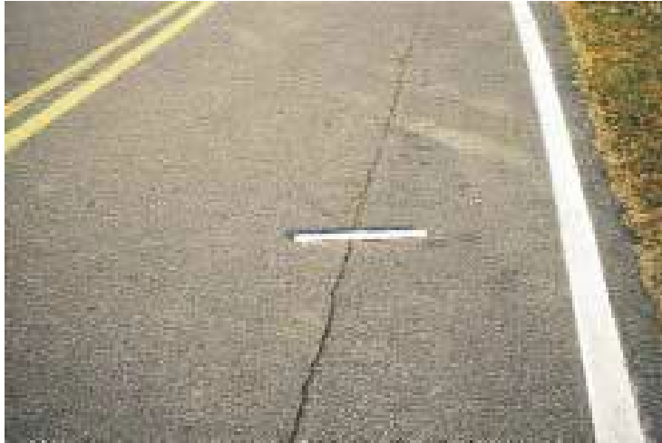
Figure 70: AC Moderate Severity Longitudinal Cracking
