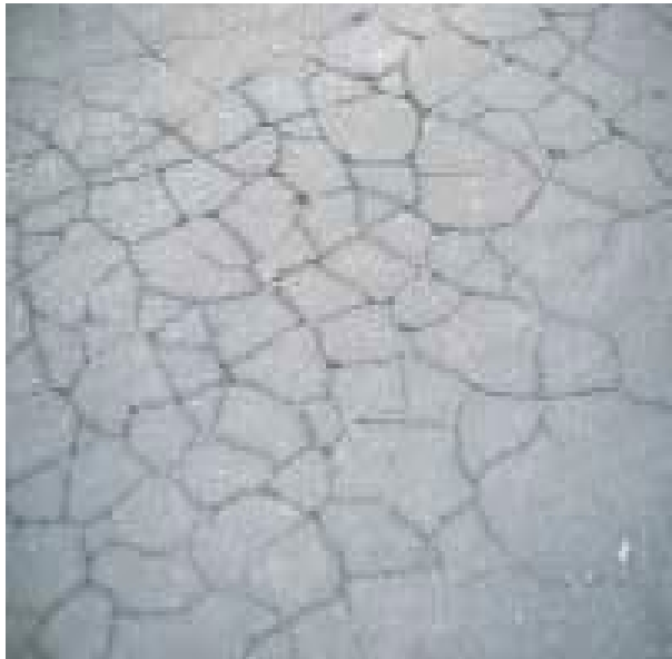
Figure 71: AC Chicken Wire/Alligator Fatigue Type Cracking
