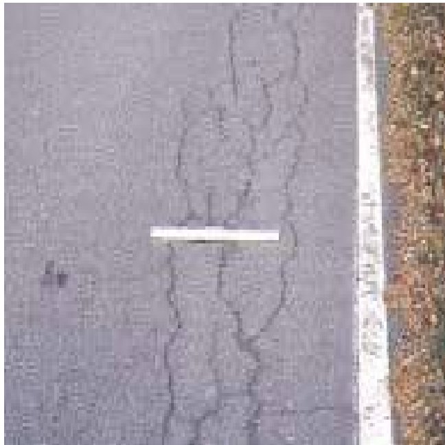
Figure 73: AC Moderate Severity Fatigue Type Cracking
