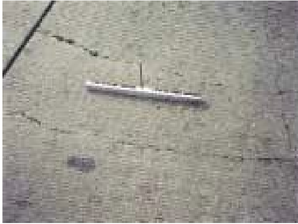
Figure 76: Low Severity CRCP Punchout Cracking
