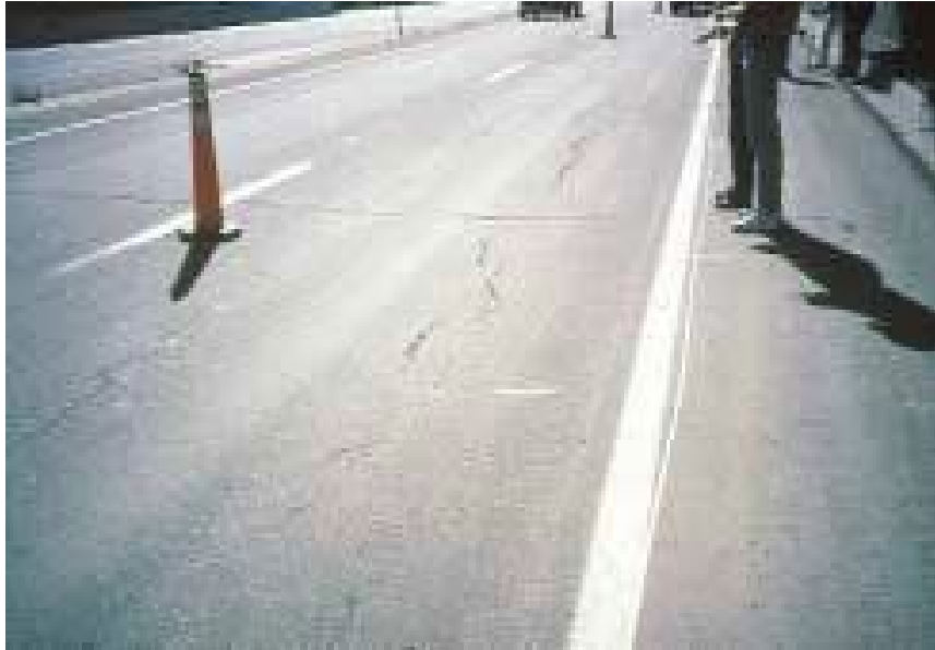
Figure 72: Low Severity Fatigue Type Cracking
