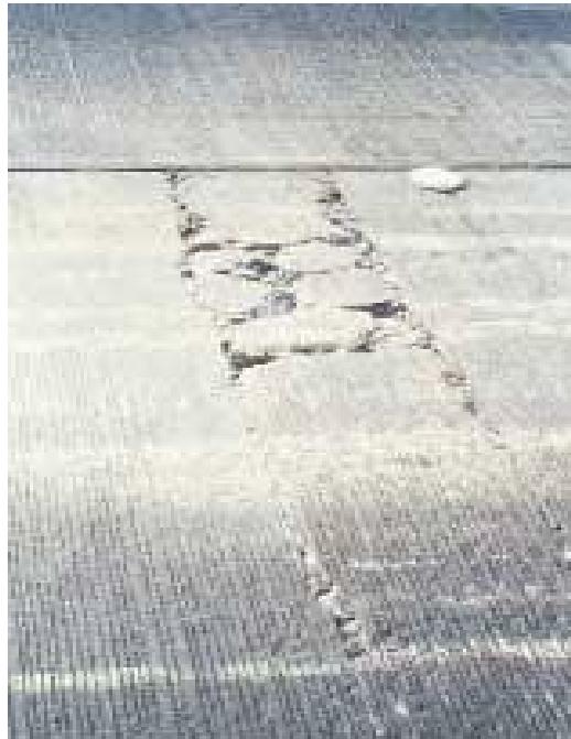
Figure 78: High Severity CRCP Punchout Cracking
