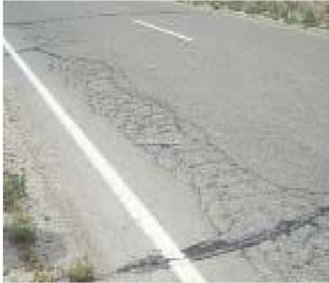
Figure 74: AC High Severity Fatigue Type Cracking
