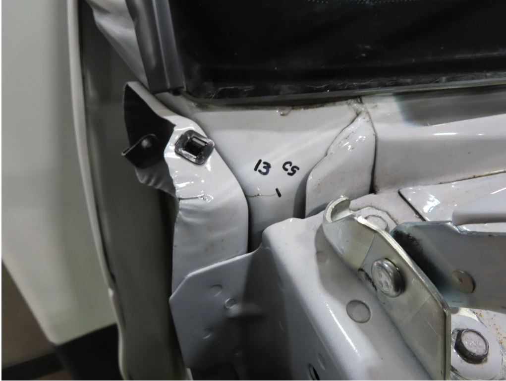
CRACK #13; CRACK JUST BELOW THE CORNER OF THE WINDSHIELD UNDER THE FENDER
