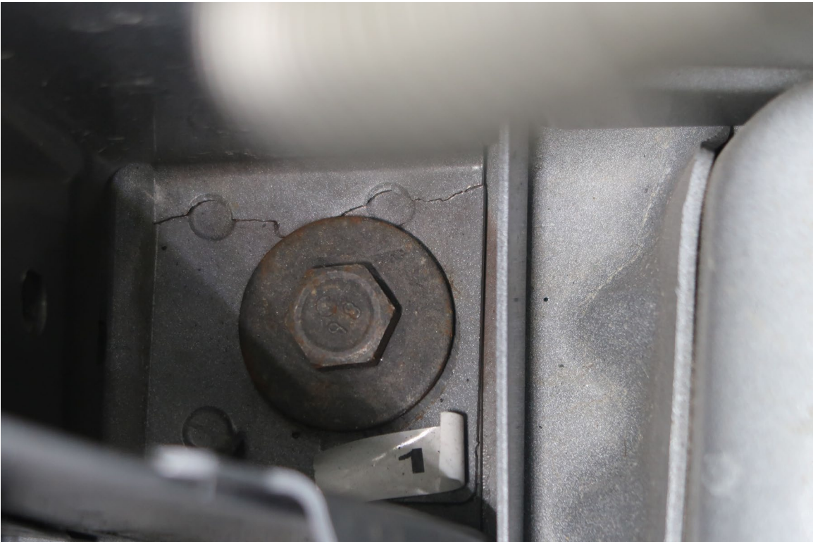
CRACK #1; CRACK ON SPOT WELDS ON THE STREETSIDE CORE SUPPORT
