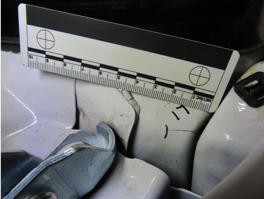
CRACK #17; CRACK ON THE STREETSIDE BELOW THE WINDSHIELD ON THE BODY UNDER THE WIPER COWL
