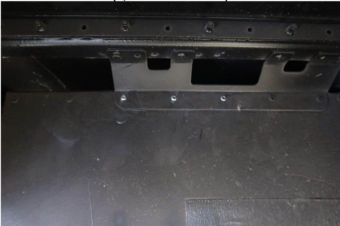
THREE RIVETS REPLACED ON REAR SIDE OF 12-VOLT AUXILIARY BATTERY BOX (2,930 TEST MILES)
