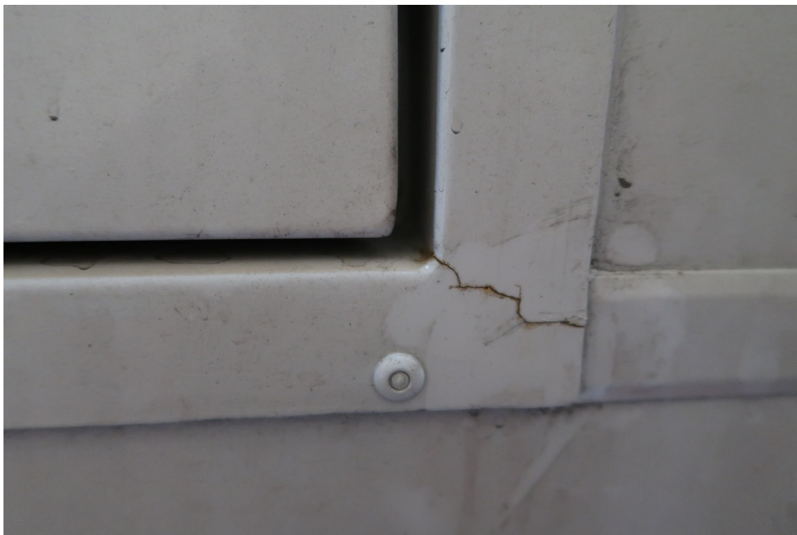
CLOSE UP OF CRACK IN THE ADA LIFT DOOR FRAME
