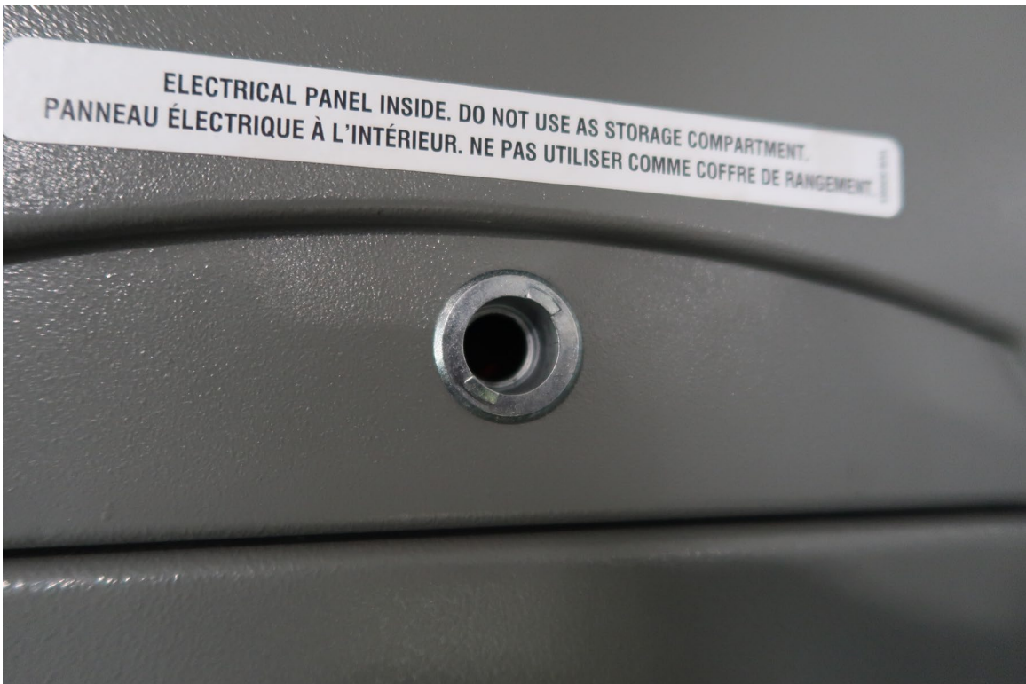
MISSING LATCH ON FUSE PANEL LOCATED ABOVE DRIVER'S SEAT (4,298 TEST MILES)
