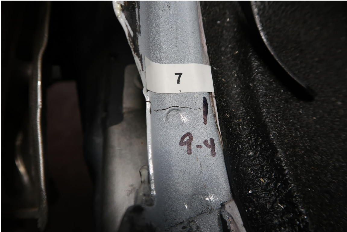
CRACK #7; CRACK ON CURBSIDE UNDER THE SEAL OF THE ENGINE ACCESS COVER
