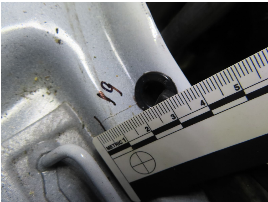
CRACK #19; CRACK UNDER THE DOG BOX
